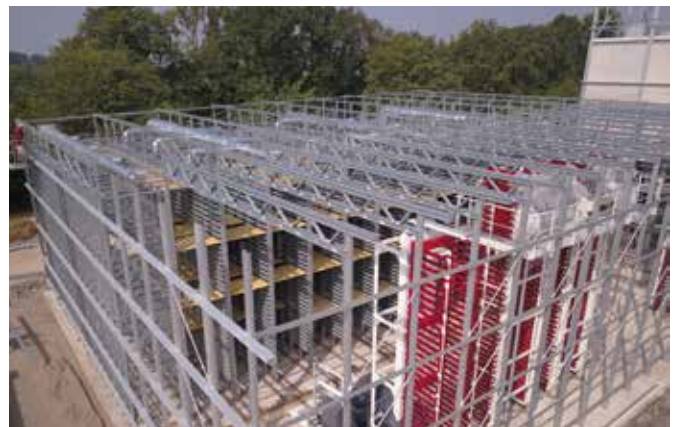
Steel construction for the vestibule of the finger car with a trussed roof girder
