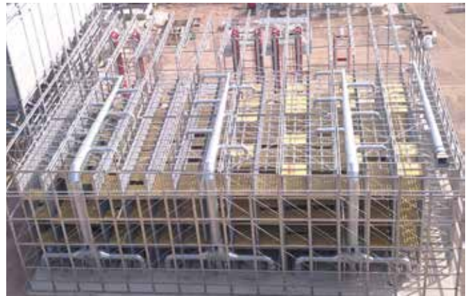
Rear view of an Outdoor Curing Chamber with the Curing System Envirocure
