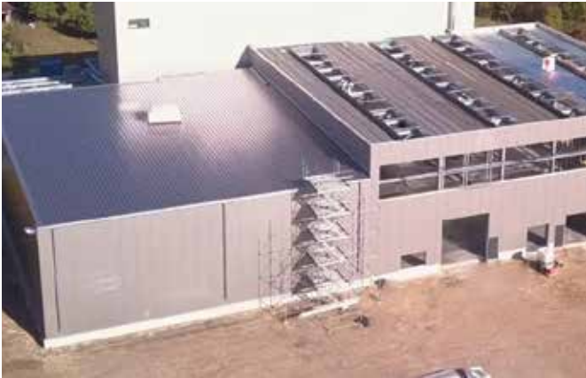
Curing Chamber cladding of an Outdoor Curing Chamber
