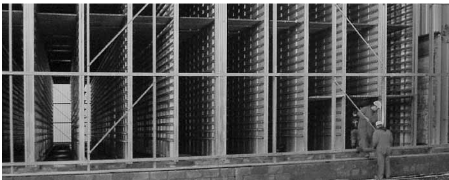
Steel skeleton of the building with curing and drying chambers; cladding takes place later – installation no problem
