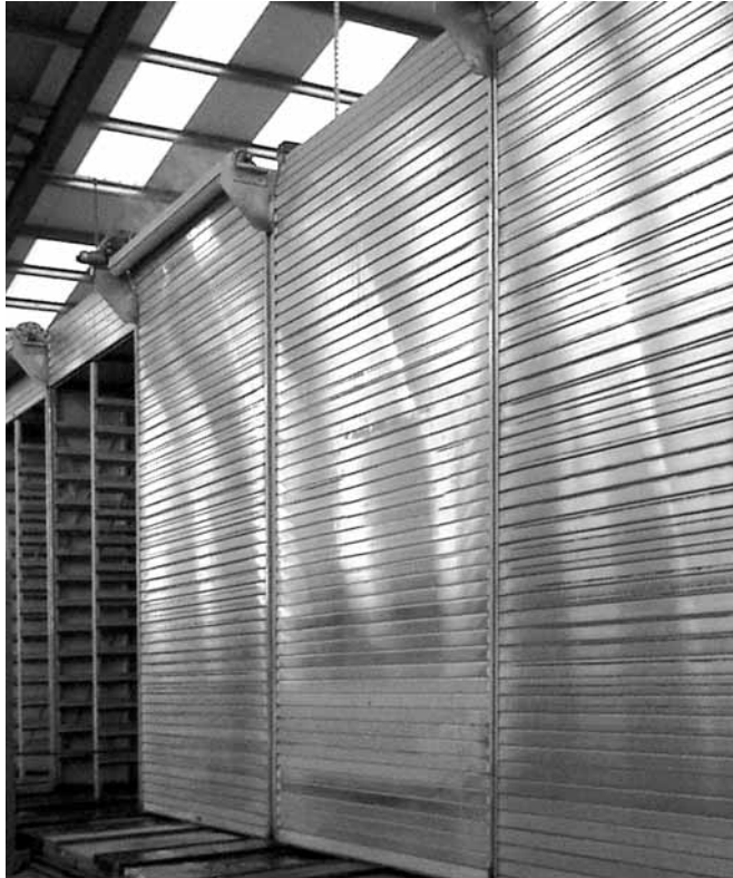
Curing chambers with roller doors is possible anytime
